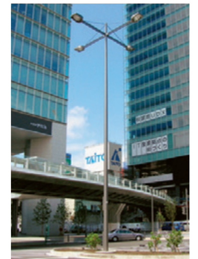
照明単独柱 Lighting Pole
