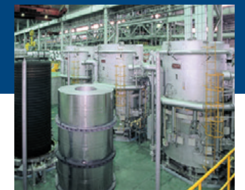
焼鈍設備 Annealing plant
