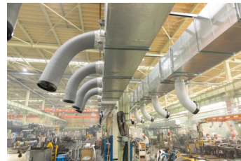
Air Conditioning Systems for Units 7 and 9 at the Tokyo Plant
